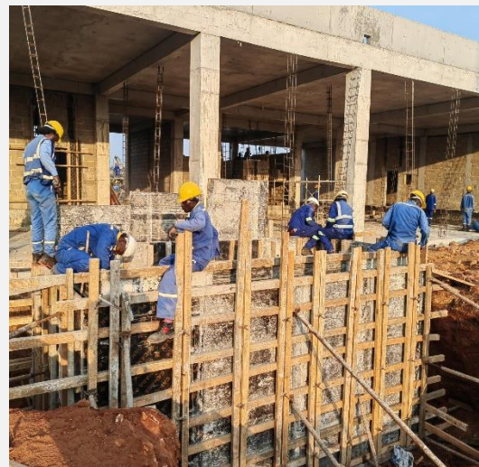
Chibuto Substation and Vilanculos Temane
