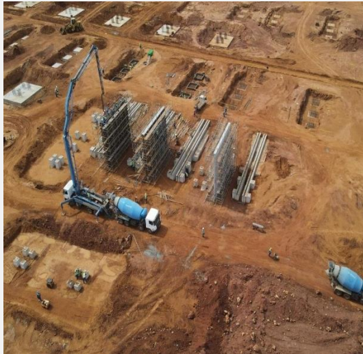
Chibuto Substation and Vilanculos Temane
